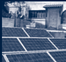
2.1 kWp PV plant fitted with ConSole
