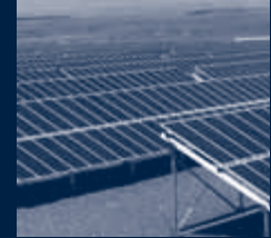
1.32 MWp PV plant near Zaragoza
