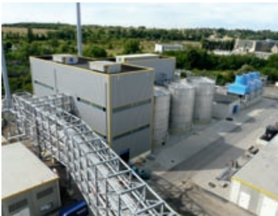
The second production line in Zeitz started production in July 2008.
