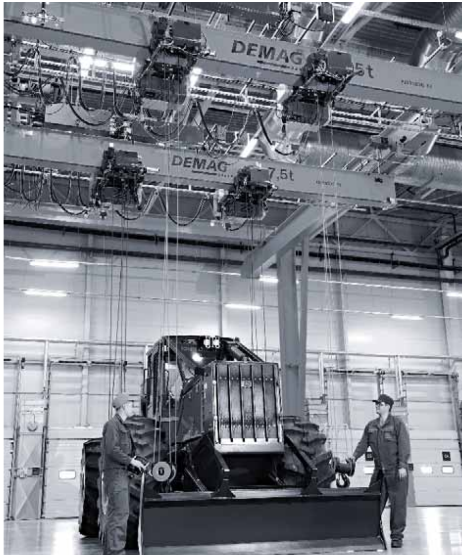
► Two Demag suspension cranes fitted with four rope hoists operating in tandem for precise and reliable handling at John Deere, Russia
