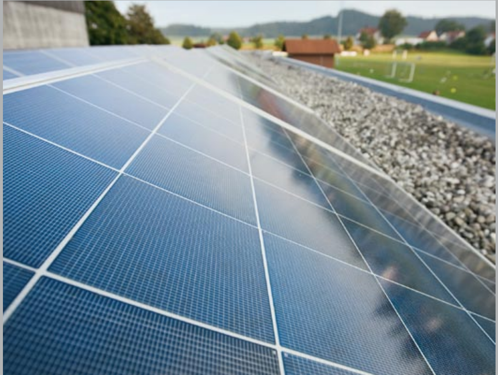
Solar panels on the roof of Aichstetten sports hall and community centre
