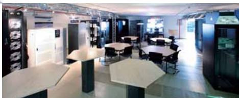
MODEL DATA CENTER IN FRANKFURT/MAIN
