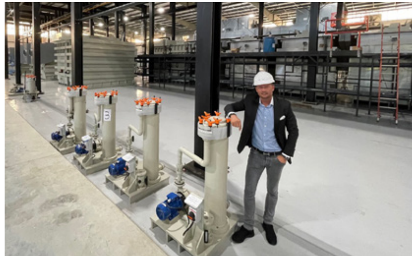
Acceptance of the new plant by the head of the KAP Surface Holding segment
