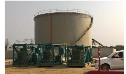
Onshore crude storage
