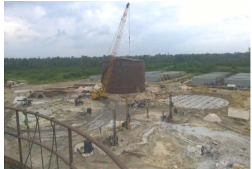
Storage Aerial View - Frac Tank 1
