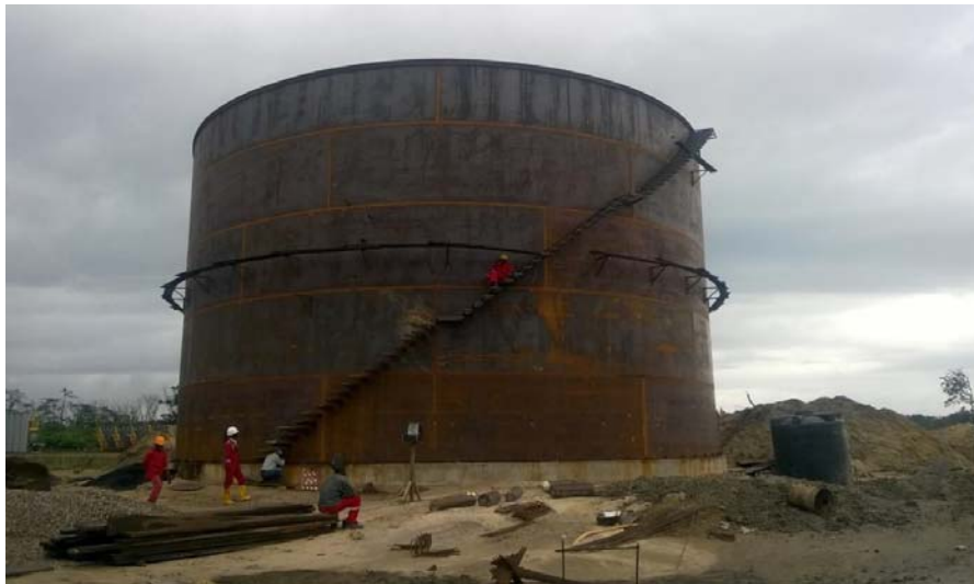
Crude Storage Tank 1
