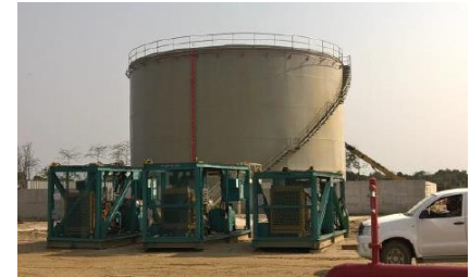
Onshore crude storage
