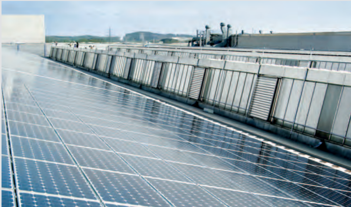
EvoBus production building, Neu-Ulm: Nearly 14,000 solar modules installed
