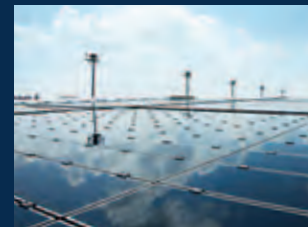
Solar power plant, Changi Airport, Singapore
