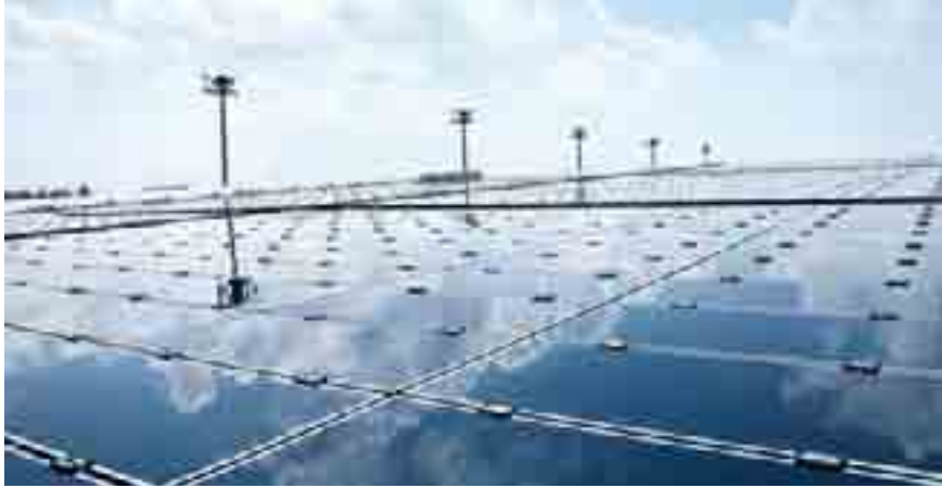
Expertise in building solar power plants – power plant built on the rooftop of Singapore’s Changi Airport.
