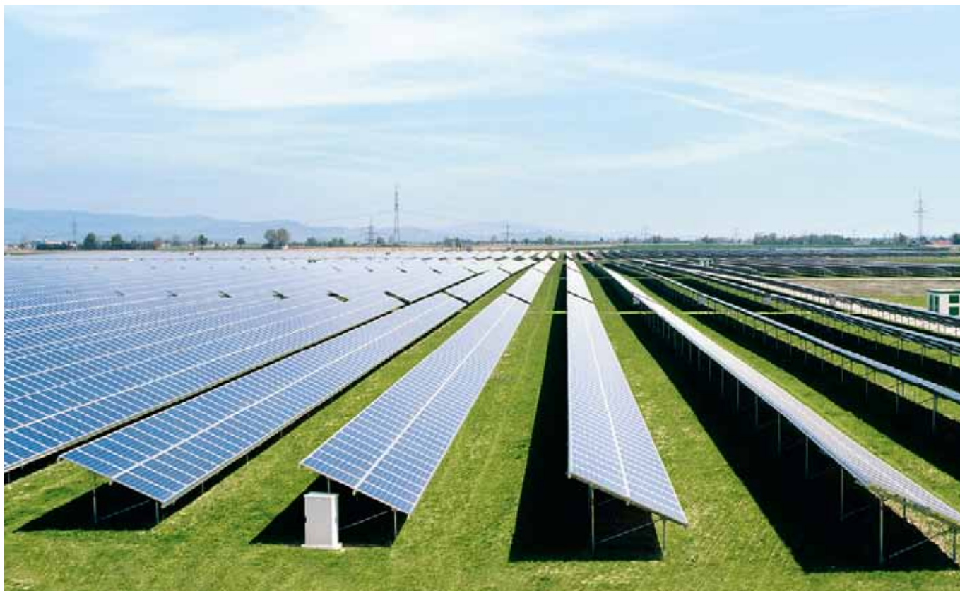
Built in record time of less than six months: the Straßkirchen Solar Park.
