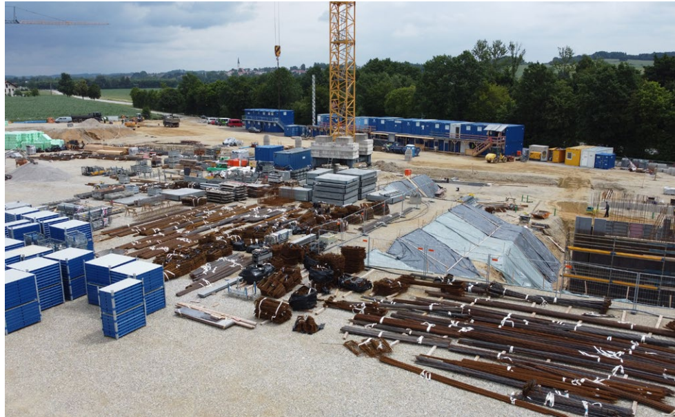
The construction of the NExT Factory in Velden to expand production capacities is fully on schedule. Production will start here in the fall of 2023.
