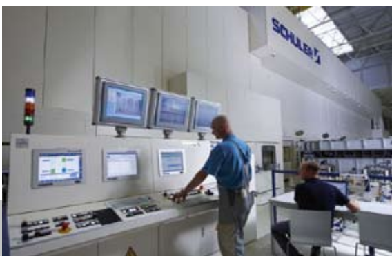
Forming processes can be easily programmed in the press line's control center
