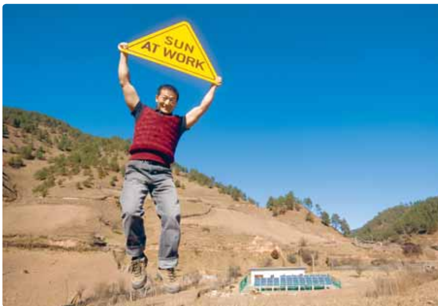
RELIABLE: 80W modules form the basis of the solar plants supplied and installed by SolarWorld. They work largely maintenance-free and – like here in Shaping – supply energy to some 40 households each.
