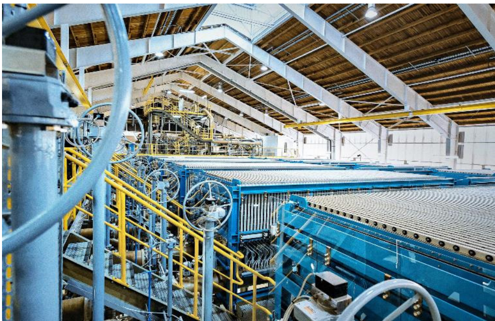
Electrolysis plant for the generation of green hydrogen
